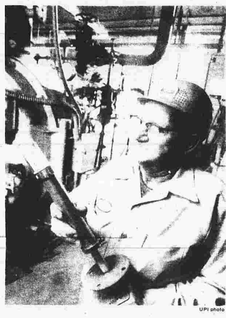
Improves efficiency Boiler operator Hurler Richter examines an oxygen analyzer which improves combustion efficiency by as much as 20 percent in small boilers like this 175-horsepower model of Dairy Form Products in Orville, Ohio. Developed by Westinghouse Combustion Control Division, the analyzer is linked to a microprocessor system which regulates air flow for combustion. Westinghouse is introducing the model this week.
